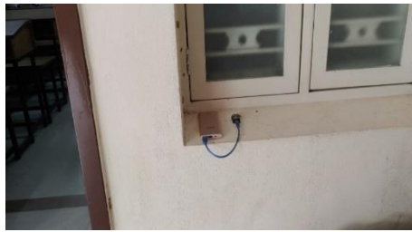
Fig.4b. XBee Router location
