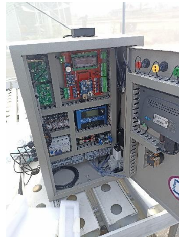
Figure 5 Hardware Control Panel
