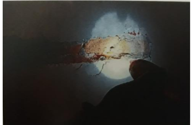
Fig 3. Cracks in the Parangkarsa Building Wall
