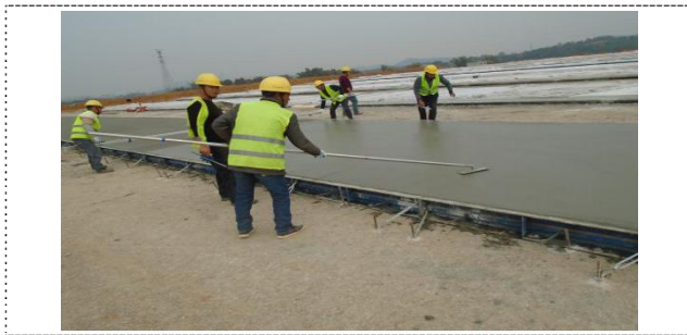
Fig. 12. Illustration of One Pass with Long-Handled Small Iron Trowel in Texture Dragging
