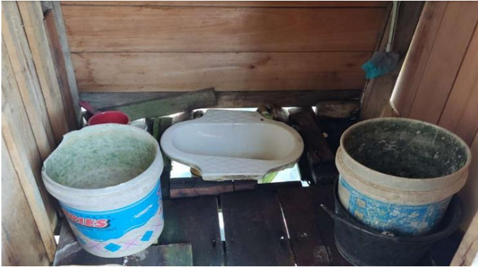
Fig. 1. Toilet without a sewage system
