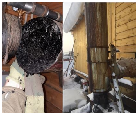
Figure 4 Left - process of soot formation in the chimney cavity of the boiler, right - process of acid condensate formation on the boiler chimney
