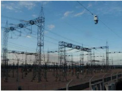
(c) Brazil substation inspection robot
