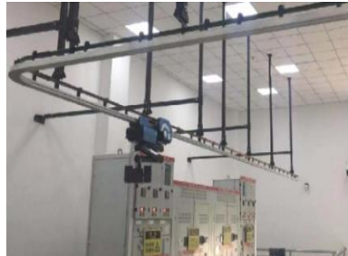
(f) China Guozi rail inspection robot
