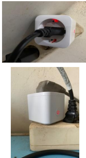
Fig. 4. Smart plug installation on TV and refrigerator.
