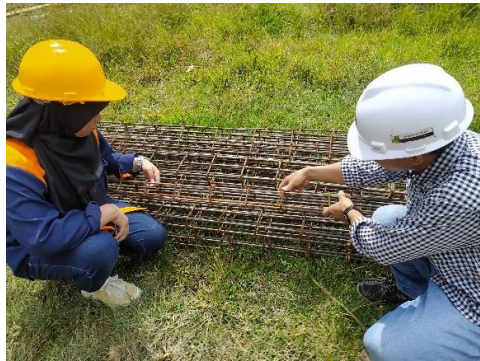
Fig 8. Column iron assembly without a 90-degree hook
