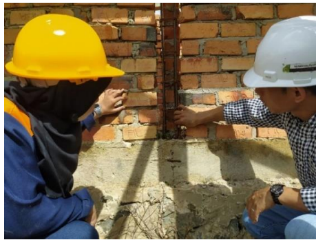
Fig 9. Building components are not connected properly.
