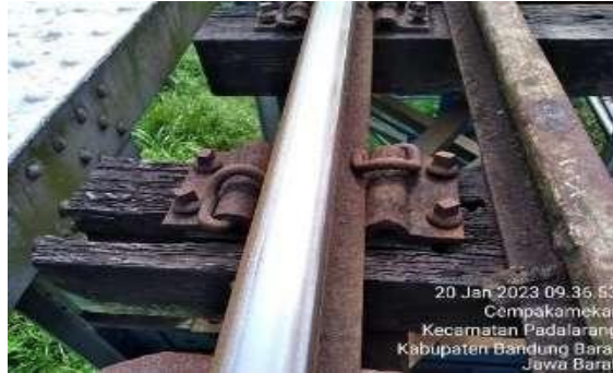
Fig. 1. Degradated wooden sleepers
