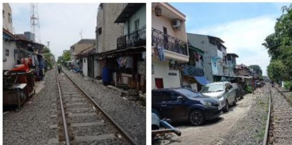
Fig. 1. Track Existing's Condition
