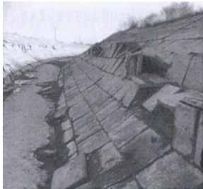
(a) Concrete slab bulge damage
