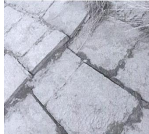
(b) Concrete slab bulge cracks
