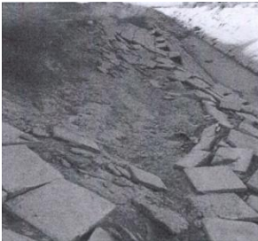
(c) Concrete slab slide
