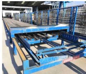
T-beam top-flange reinforcement skeleton tying by unit frame (b) unit reinforcement moulding frames
