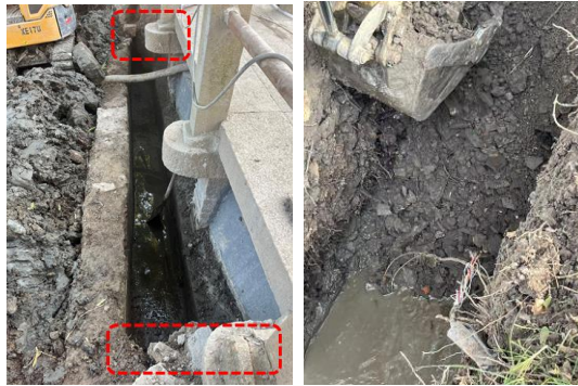
Fig. 7. Leakage location and situation
