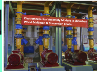
Fig. 17. Modular equipment room
