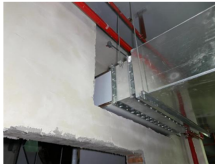
Fig. 7. Reserved mechanical and electrical holes
