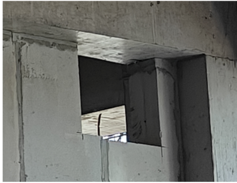
Fig. 8. Reserved mechanical and electrical holes
