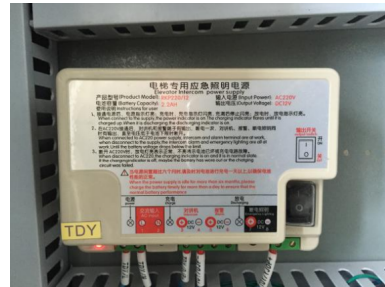
(b) control cabinet
