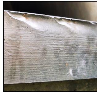
Fig. 2. Grooved erosion on the upper edge of the lower ring of Unit 1#
