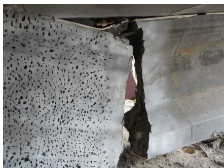
Fig. 7. The destruction of the experimental beam
