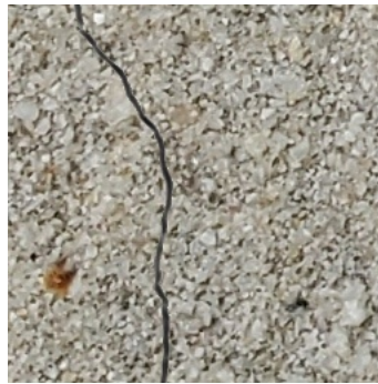
(c) Cracks on concrete background (using style transfer technique)
