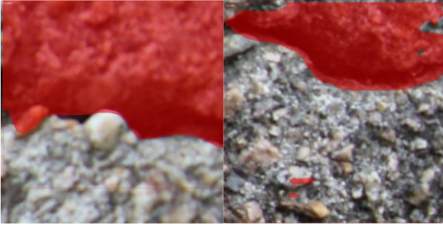
Fig. 15. Image elimination based on the crack width anomaly
