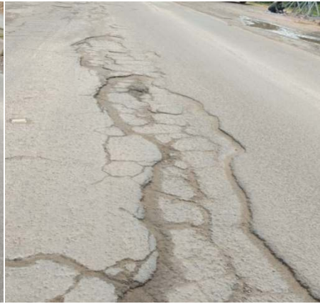
Fig. 2. Fatigue of pavement along the length.
