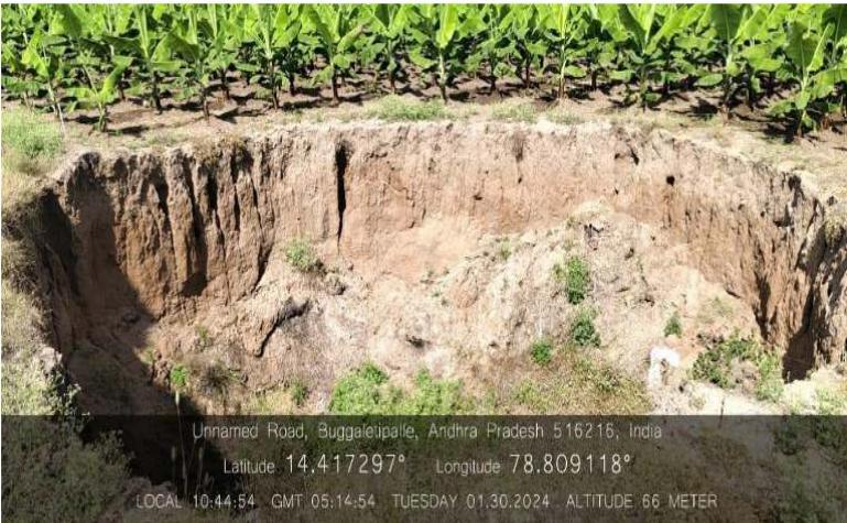
Fig 4. Geotagged location of the sinkhole-formed area
