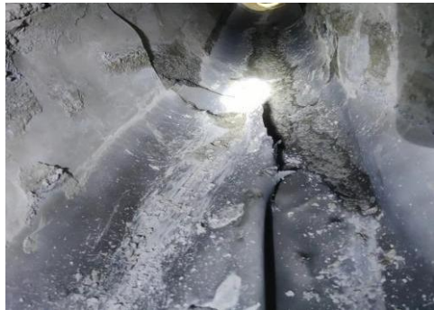
Fig.7. Waterproofing sheet breakage
