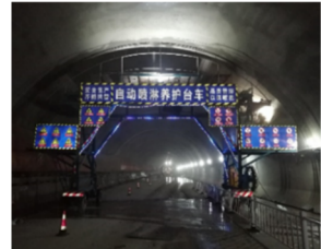
(f) Automatic spray maintenance trolley
