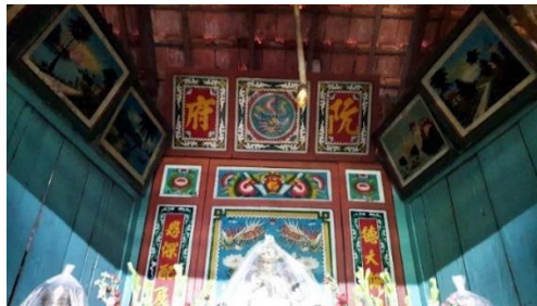
Fig. 16. Altar paintings and decorative paintings are arranged above the altar room in contact with the tiled roof. (Source: Author, 2020)
