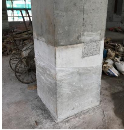
Fig. 17. Effect of Concrete Column Bottom after Mold Removed
