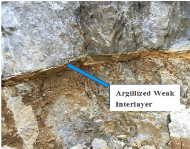
Fig. 2. Argillized Weak Interlayer.
