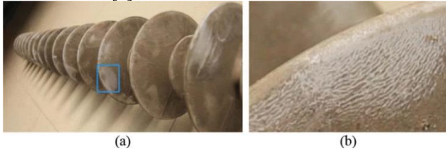
Fig. 1. Micro-cracks on an insulator [6]
