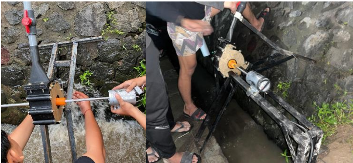
Figure 7. Turbine Set Up with Small Generator
