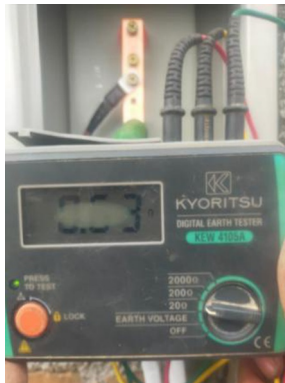
Figure 2. Results of Ground Resistance Measurement Using the Kyoritsu 4102A Earth Tester
