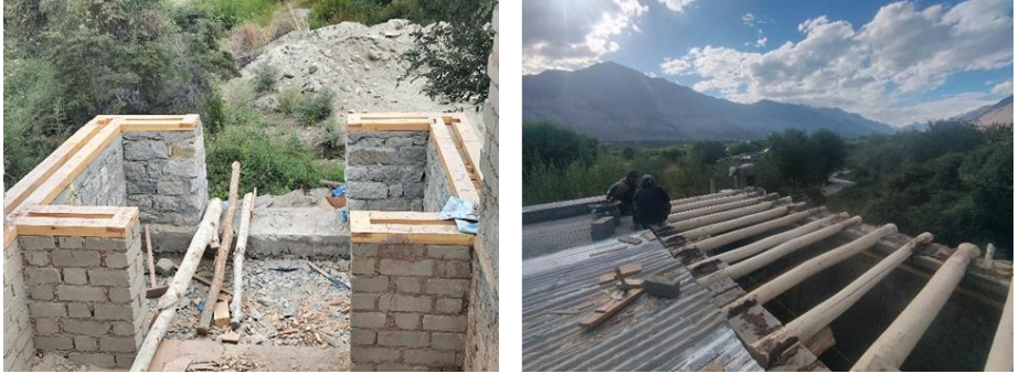
Fig. 11. Timber runners at sill level in taq construction (left); Wooden beams to transfer load and enhance box nature of structure (Right)
