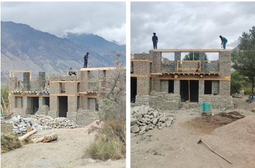
Fig. 10. North Indian builders use taq techniques for modern construction projects throughout the region.
