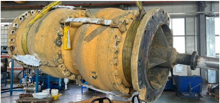
Fig. 1. Severely Consumed Sacrificial Anode from Electrical submersible Pump
