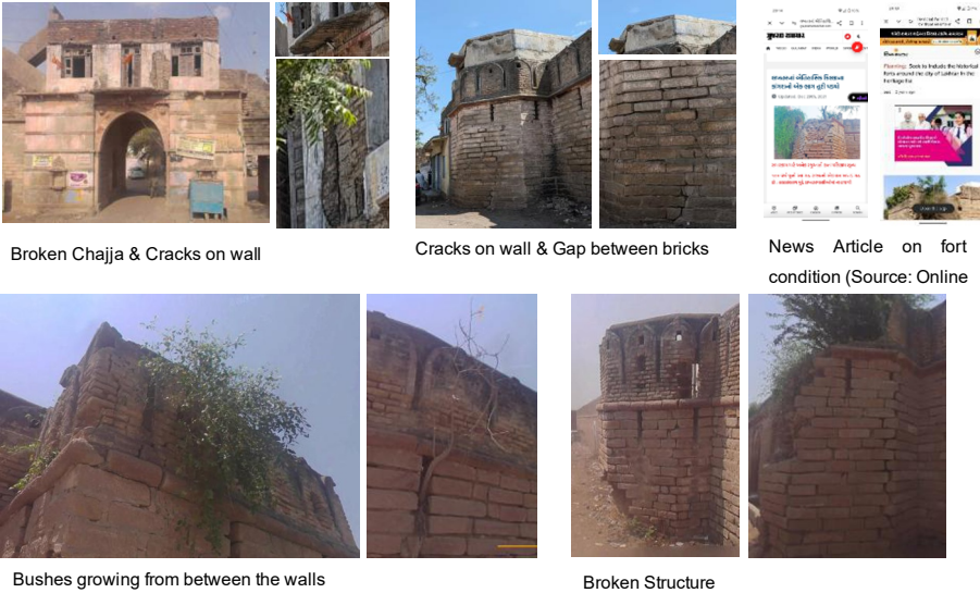
Fig.35. Images highlighting the deteriorating condition of for
