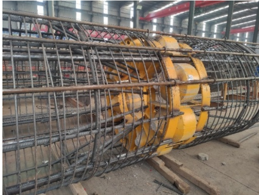
Fig. 1. Schematic Diagram of the Load Cell and Its Connection to the Reinforcement Cage in the Test Pile
