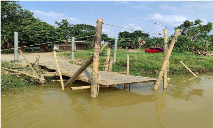
Figure 1.1 condition of the Rowosari-Yosorejo pier
