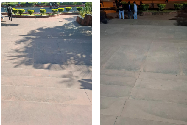
Fig. 7. Staircase Visibility Deficiency Due to Lack of Edge Contrast Source: Author.
