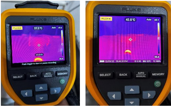
Fig 6. Thermal image sensor shows the temperature at different locations of casing
