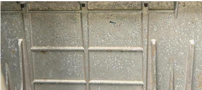
Fig. 1. White rust observed in aluminum casing
