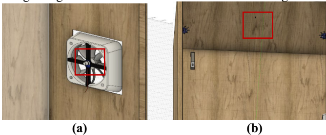
Figure 6. (a) MQ-2 Smoke Sensor Position. (b) LM35 Temperature Sensor Position.
