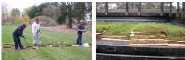
Figure 4 Lifting the cut sod onto boards using a shovel (left photo) and stacking the boards for transport on a trailer bed (right photo).
