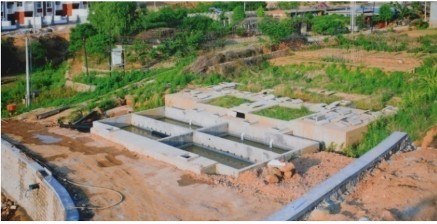
Figure 1. No powered sewage treatment system.
