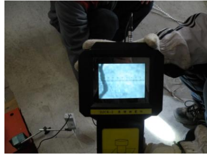
Fig.2 Crack width measurement
