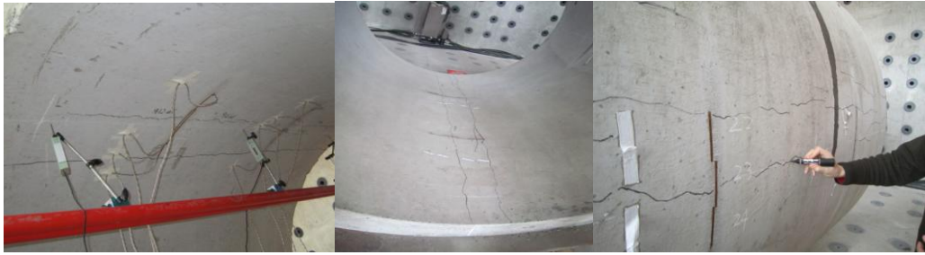
Fig.7 Crack distribution shown
