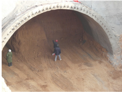
Fig.5 Excavation method in portal section supported by leading pipe-shed in loess tunnel
