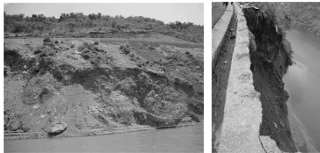
Fig.1 Site photograph for landslide in the reservoir
