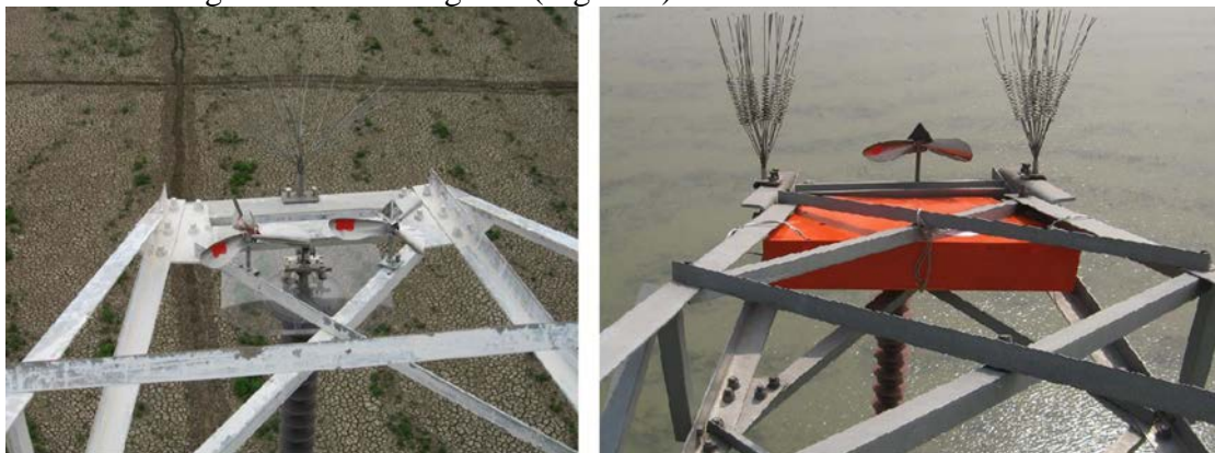
Figure 2 bird excrement flashover prevention measures
