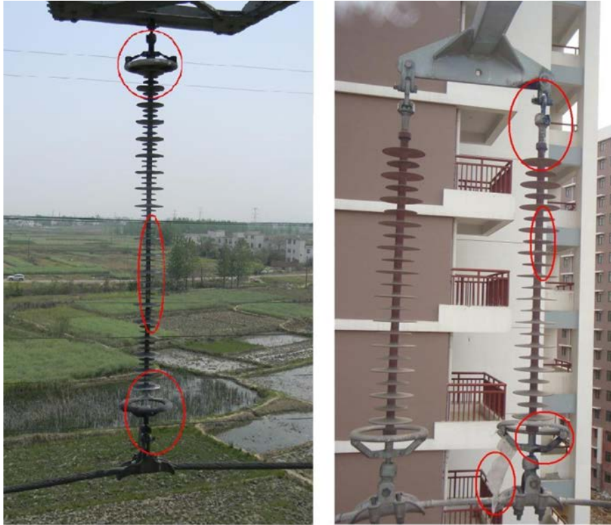
Figure 3 comparisons between bird excrement flashover and foreign body flashover
