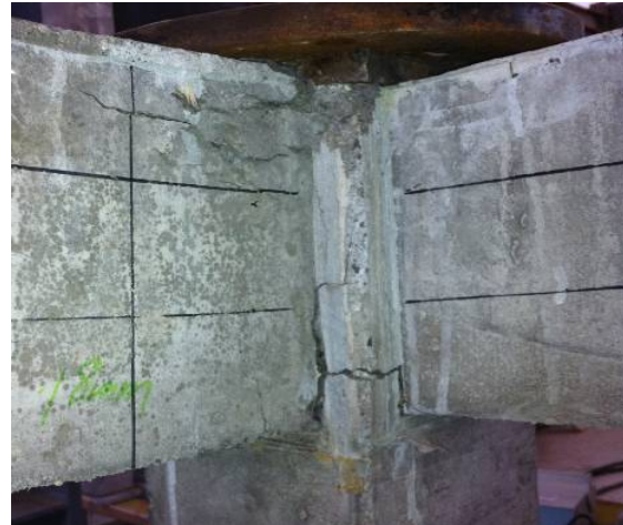
Fig. 4. In condition S2, cracks of settling column-beam joints
