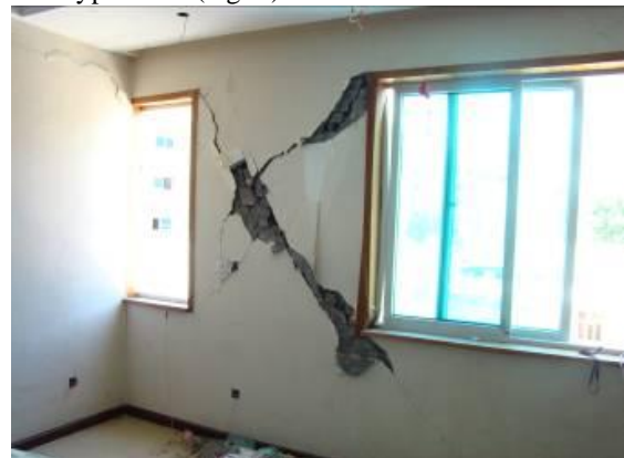
(a) Inclined cracks in wall between windows(internal).
