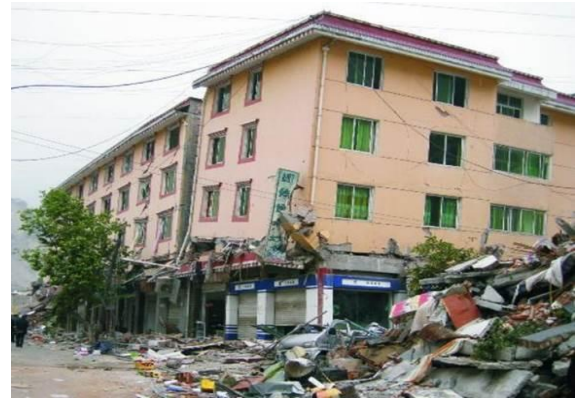
(a) Damage of the transition layer.
