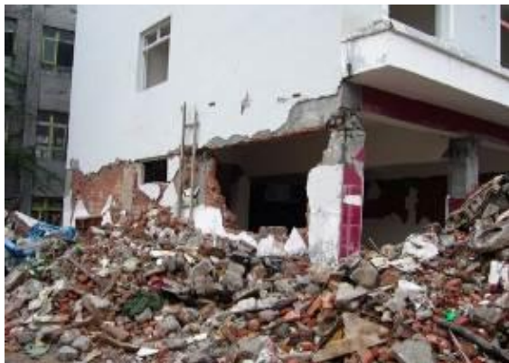
(b) Damage of masonry anti-seismic wall in horizontal direction.
