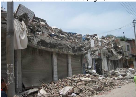
(a). Collapse of upper masonry layers.
