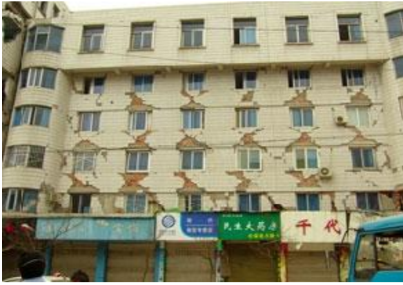
(b) Damage of the wall under windows in upper masonry layers.
