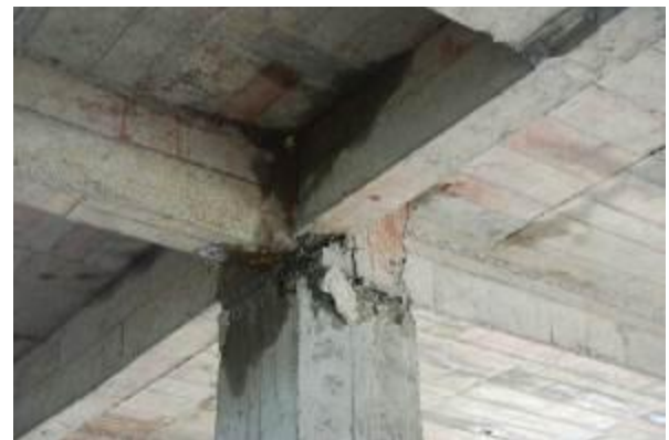
(b) Plastic hinge appears in beam-column joint.
