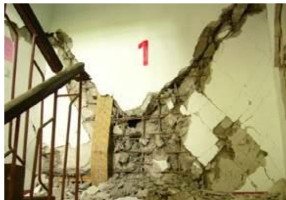
(a). Shear failure of reinforced concrete anti-seismic wall.
