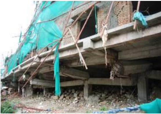
(b) Collapse of the bottom layer.
