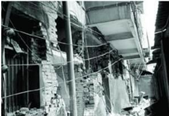
(a) Damage of masonry anti-seismic wall in longitudinal direction
