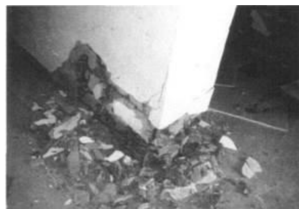
(b). Damage of wall corner.
