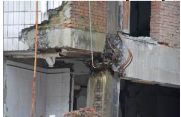
(a) Compressional buckling of steel bar of column.
