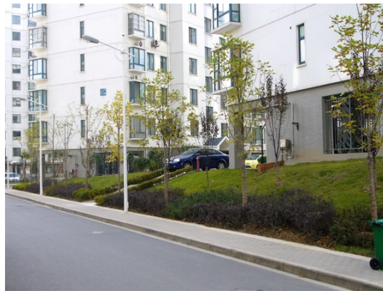
Fig. 1 Subsided Building Apron of Yu Yuan residential quarter
