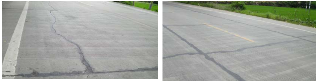
a.Longitudinal cracks b.Transverse cracks Figure 1 Disease chart of cement concrete overlay
