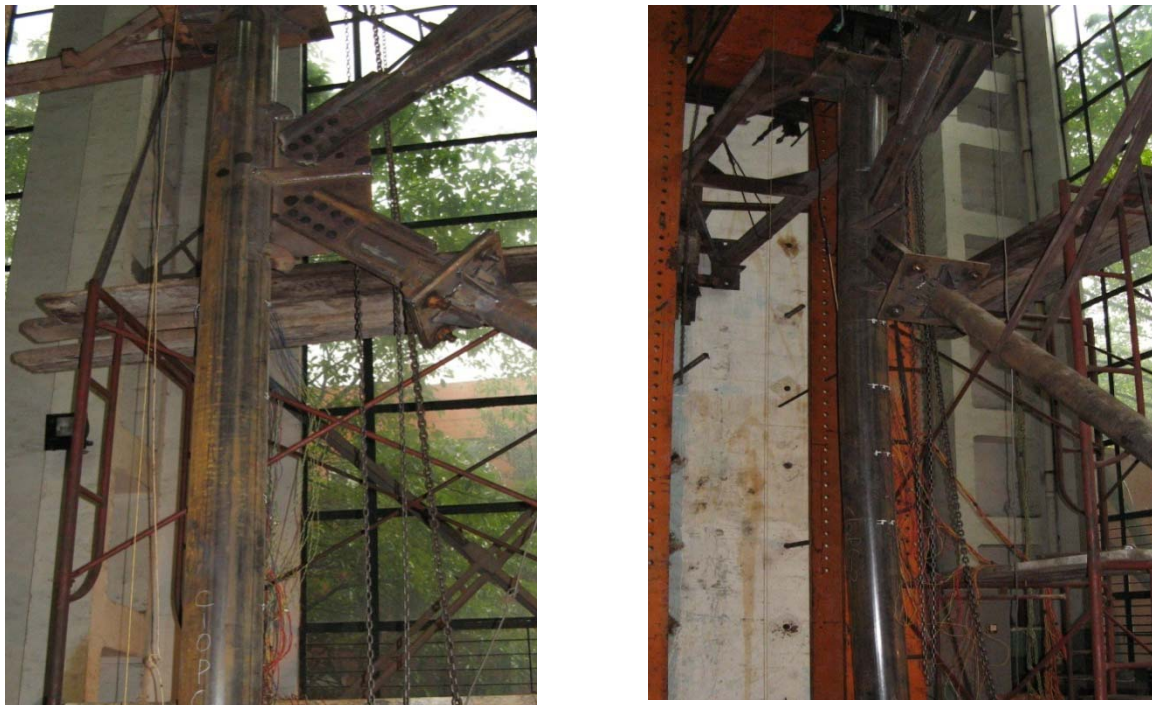
Figure.4 C1PC Failure Form
