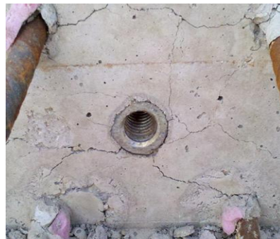
2 Stress crack Fig.
